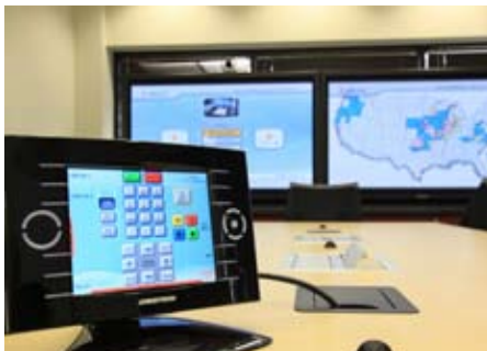
crestron control in video conferencing room
