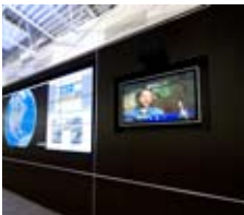
network operation center
