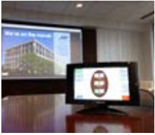
Crestron room control
